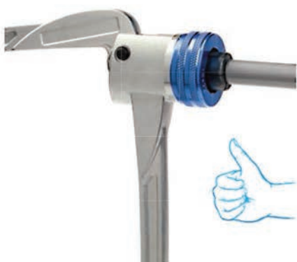
▲ Fig. 30: Pipe until end of expander.
